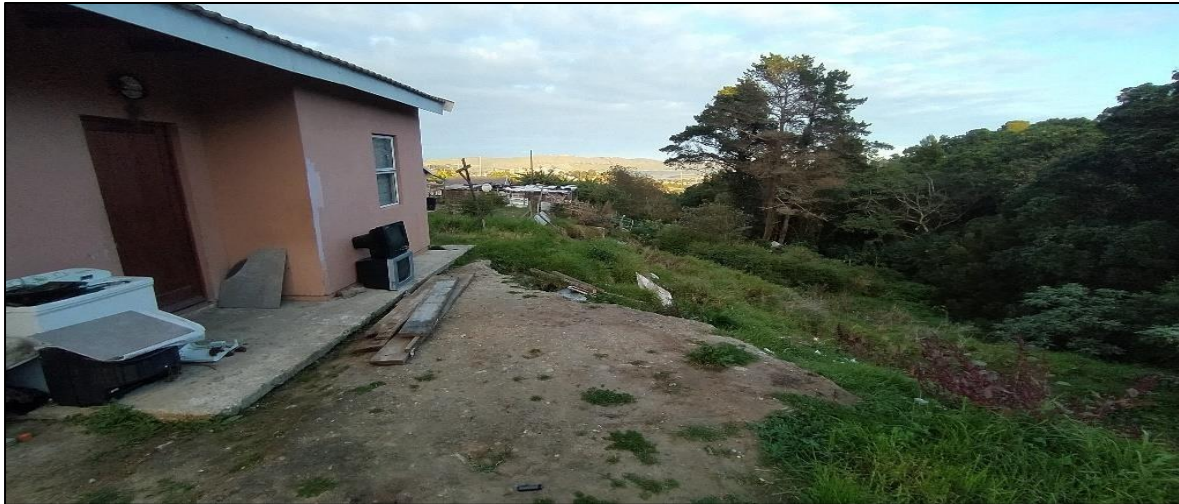
Soil erosion closer to the Bongani stream
