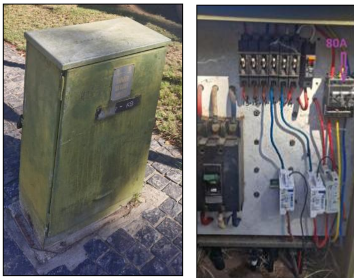
Fig. 3&4) Street kiosk fed from MS in Heron Street providing 60A 1ph to houses and 80A 3ph to the church building
