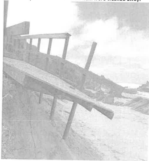
End of boardwalk. Most of the boardwalk was completely washed away.
